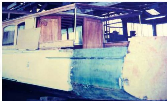
Restoration and extension, 1994-95; above, with the old stern cut away, and below, with the new extension welded into place
