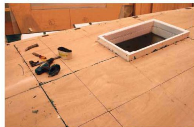
Two views of the ply sub-deck. Would the old boatbuilders have used ply if they could? Probably – it helps stiffen and waterproof the boat
